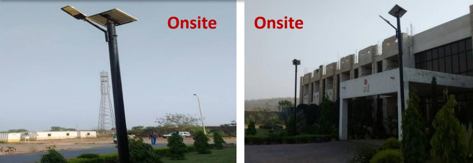
PV Solar Street Light Inside Plant
