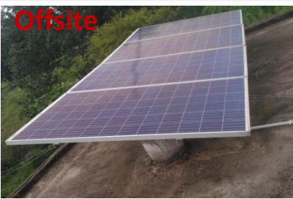
PV Solar Panel Installed at Intake Pump House
